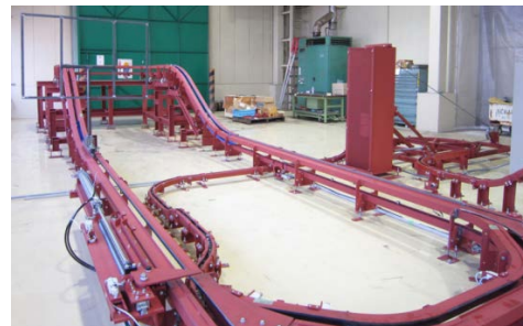
Conveyors for transporting lightweight items for car manufacturers
