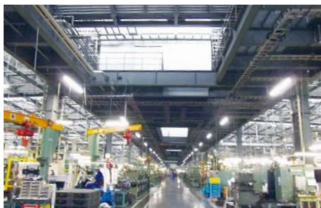
The main factory building after changing over to 200 LED lights
